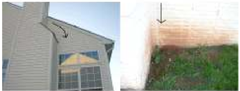
Settling from Roof Runoff
