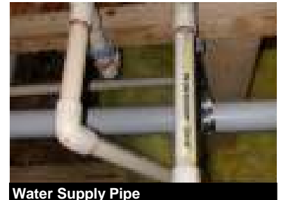
Water Supply Pipe
