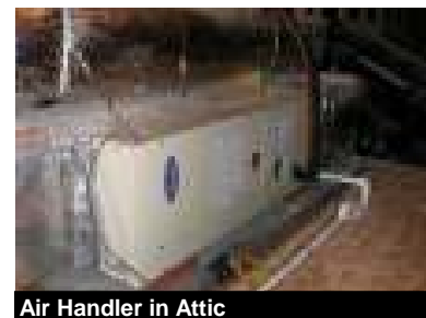
Air Handler in Attic
